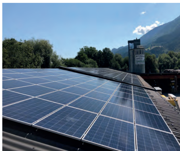
Photovoltaikanlage Fa. Pitzer & Huber
