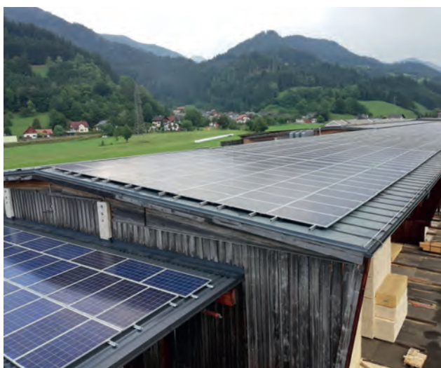
Photovoltaikanlage Fa. Kaml & Huber, Bärndorf
